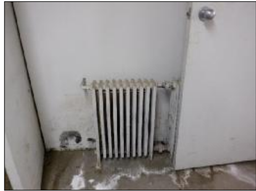
Interior, As-Is – basement, radiator
