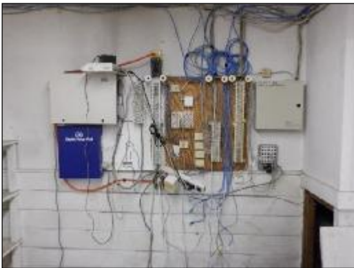
Interior, As-Is – basement, communications
