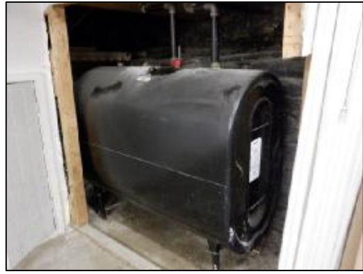
Interior, As-Is – basement, oil AST
